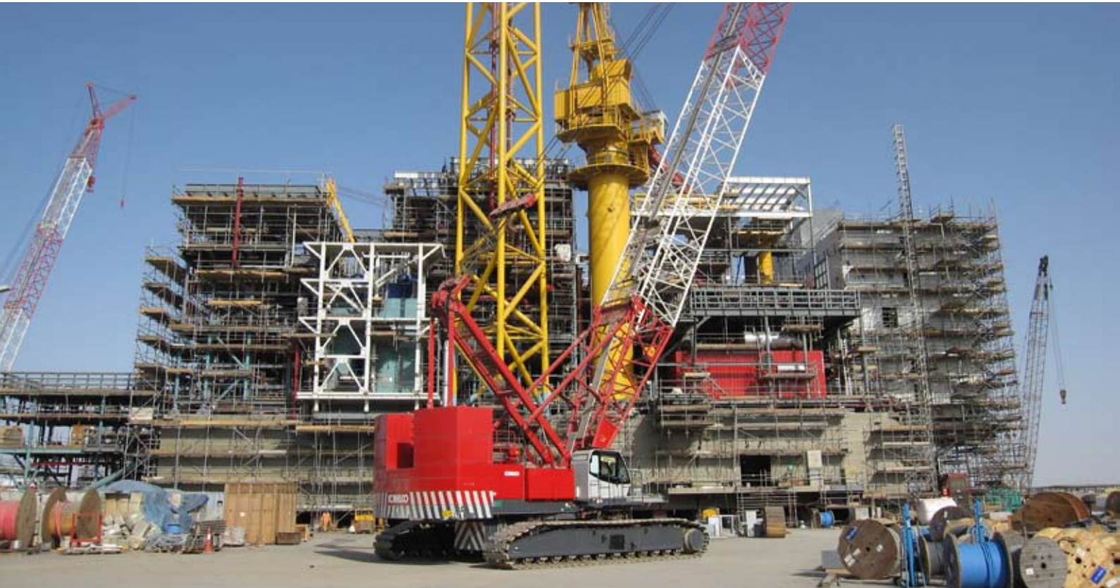
MOPU at Ad-Yard: Outboard Staircase, DOP's & Bumper Bars on Weather Deck, lower half flare stack
